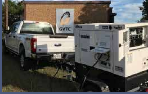
USA, TV relay station
